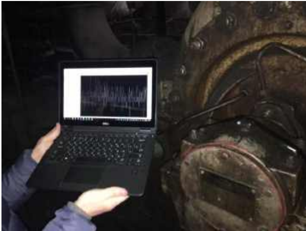
Figure 2 – Functionality testing of a laboratory prototype of a wireless vibration diagnostics system for power generation equipment at the Darnytsia CHP
